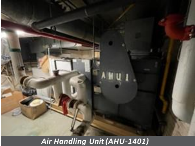
Air Handling Unit (AHU-1401)
