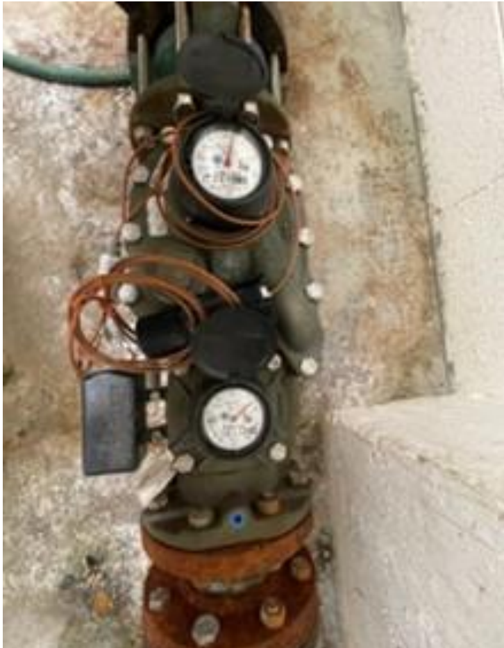
Fig. 3 Building Water Meter
