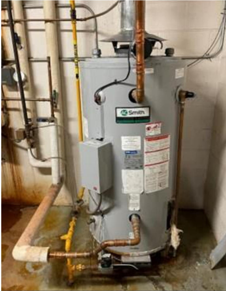
Fig. 4 Natural Gas Hot Water Heater
