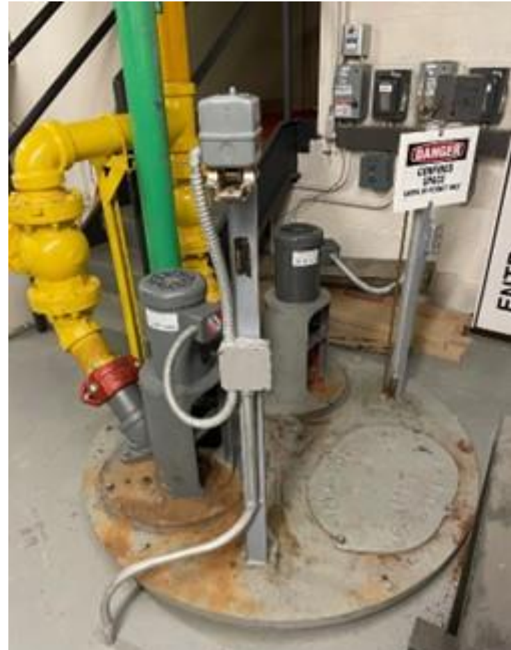
Fig. 6 Sewer Ejector Pumps (1416, 1417)
