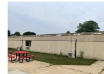
McNeel - Synthetic Stucco Degradation and Fascia Damage
