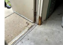
McNeel Exterior Door Frame Damage
