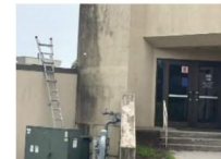
McNeel - Synthetic Stucco Moisture Damage
